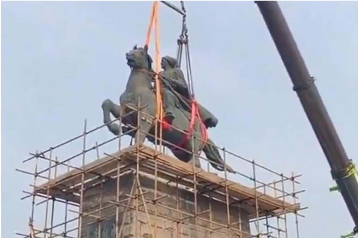
Figure 10: Removal of the statue of Li Zicheng from Beijing in May, 2024 The statue was too frightening for the regime.
